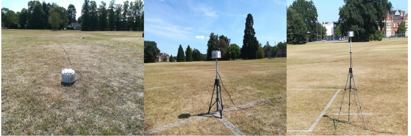
Fig. 8. Photos about the installation of the BOLTEK EFM 100 field mill at different heights (15 cm, 1 m and 1.8).
